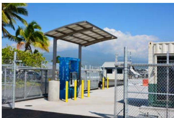
Figure 4: NELHA Hydrogen Station Dispenser
