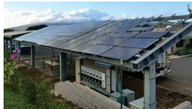
Fig. 1: PV test platform commissioned in February 2016 in Kihel, Maui. Lat: 20.7°N, Long: 156.4°W, Alt: 60 meters, Tilt: 20°, Azim: 197°N
