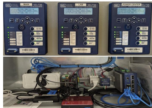
Figure 1. SEL-735 power quality meters (top) and communication interface (bottom) configured at the NELHA Research Campus.
