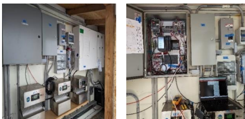
Figure 1. DC microgrid components in the electrical room (left) and system's controller box (right).
