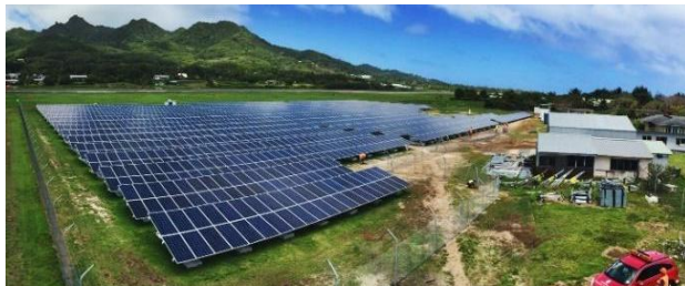
Figure 1. Te Mana o Te Ra PV + BESS Project (1 MW, 5.6 MWh) at Rarotonga International Airport.
