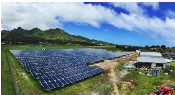
Figure 2. Te Mana o Te Ra PV + BESS project (1 MW, 5.6 MWh) at the Rarotonga International Airport.
