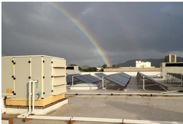
Figure 2–23 LDAC unit and solar system at Whole Foods Market, Kailua, Hawaii (Credit: Ian Doebber/NREL)
