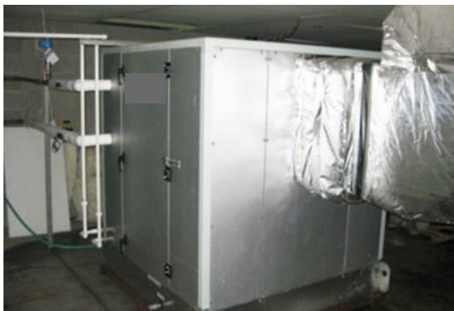
Figure 2–52 LDAC conditioner in the mechanical room of the Babbio Center (Credit: AIL Research, with permission)
