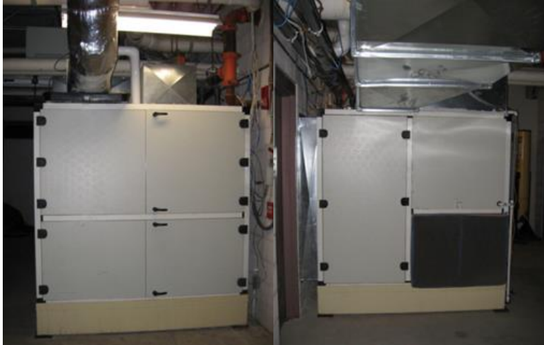
Figure 2–42 LDAC unit in the basement of the Schaefer Pool facility (Credit: AIL Research, with permission)
