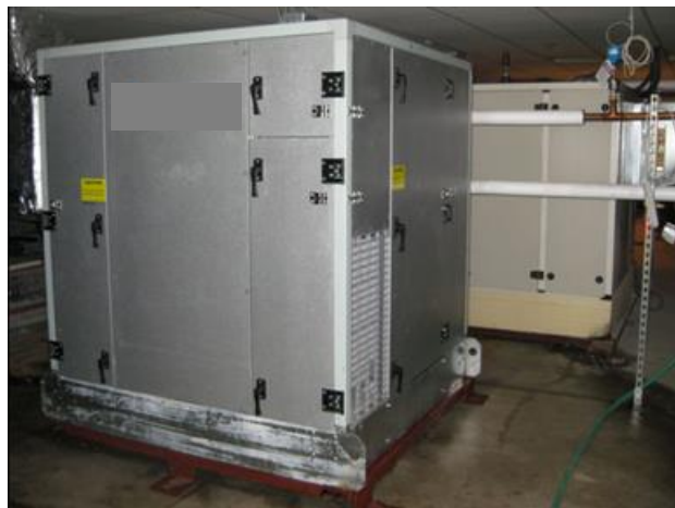
Figure 2–51 LDAC regenerator and conditioner in the mechanical room of the Babbio Center (Credit: AIL Research, with permission)
