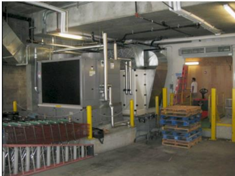
Figure 2–6 LDAC and chiller system in loading dock at Whole Foods, Encinitas, California (Credit: Jeff Miller/AIL Research, with permission.)
