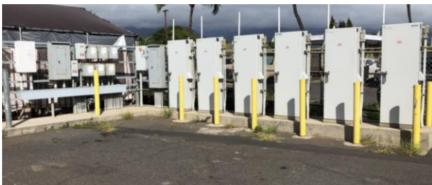
Figure 1. Sunverge Solar Integration System (SIS) BESS + PV units.
