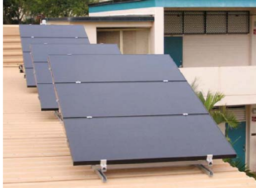
Figure 1: HECO 2 kW "SunPower for Schools" PV installation at Jarrett Intermediate School comprising 10 mono-crystalline silicon panels
