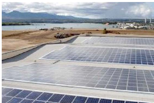
Figure 2: The Navy's 300kW Ford Island PV installation comprising 1454 poly-crystalline panels
