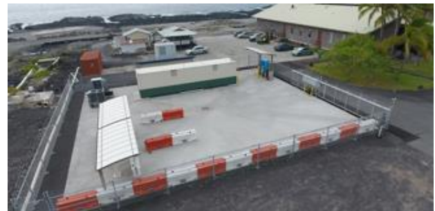
Figure 3. HNEI Hydrogen Station
