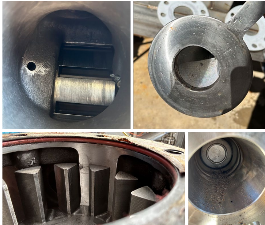
Figure 8. Feed pump damage.
