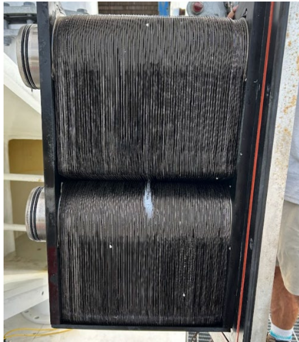
Figure 13. White residue at the center of the stack is indicative of an ammonia leak.
