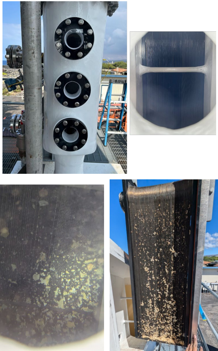
Figure 12. (top) View ports installed to monitor evaporator leading edge. (bottom) Debris from seawater piping system collected at the evaporator leading edge as seen through the viewport and when evaporator was removed for cleaning.
