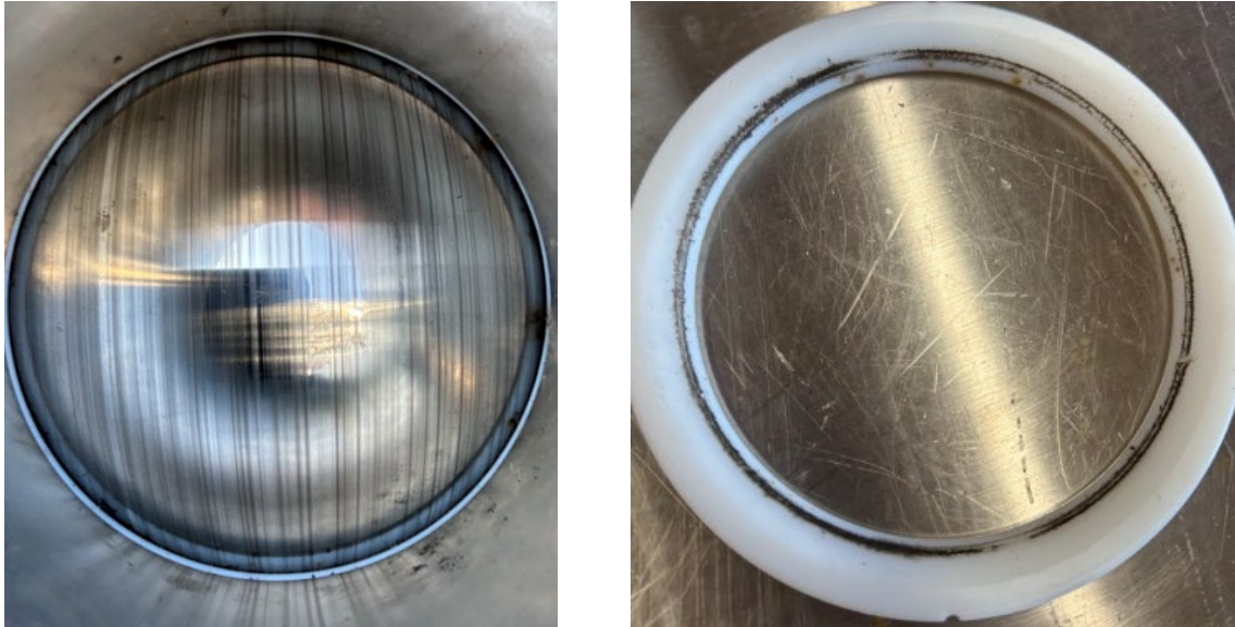
Figure 11. Weld slag in valve seating surfaces prevent quick-close valve from sealing.
