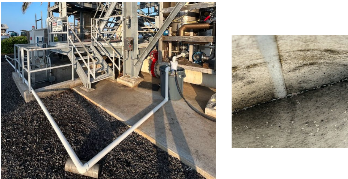
Figure 10. Flushing the ammonia line between the feed pump outlet and recirc pump inlet did not remove significant amounts of shavings/debris.
