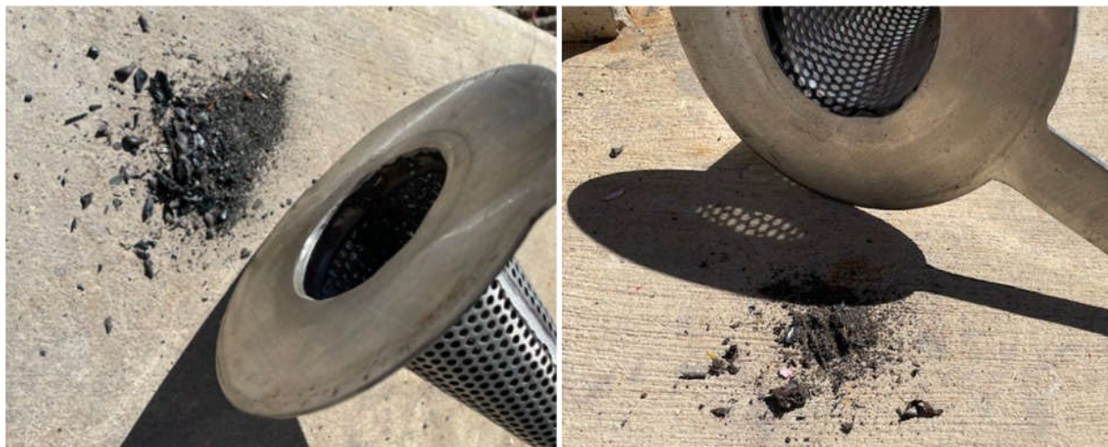
Figure 6. Debris in ammonia piping caught in strainer.
