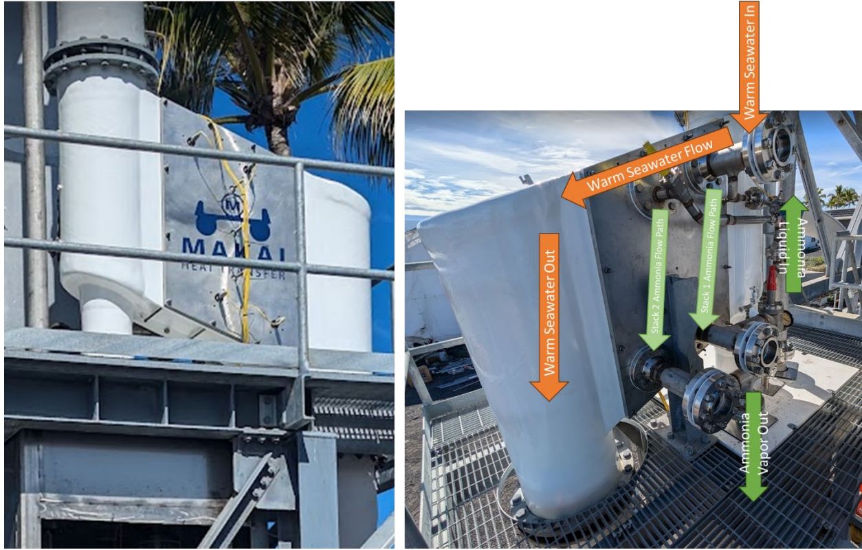
Figure 4. Evaporator installed in HX Tower
