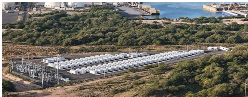
Figure 4. Example of a typical battery bank.
