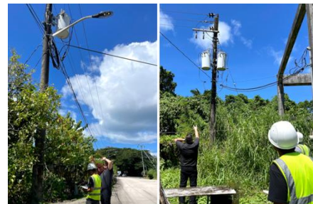
Figure 2. Grid START and PPUC personnel conducting a field survey of transformers.
