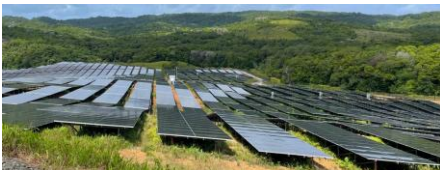
Figure 1. PV arrays at Palau's SPEC PV+BESS plant.
