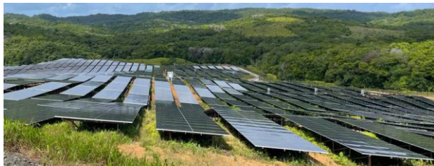
Figure 1. PV arrays at Palau's SPEC PV+BESS plant.
