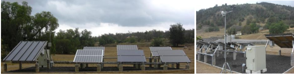
Figure 1: PWW, Kona Coast of Hawaii – PV systems ground mounted on open rack structures (left) at the bottom of the Puu Waa Waa hill (right)
