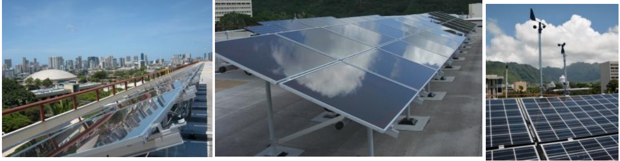
Figure 9: GHHI, Honolulu, Oahu – PV systems mounted on open rack structure (middle) located on a flat roof on the Koolau Range Mountain slope (background, right image) overseeing Honolulu (background, left image)
