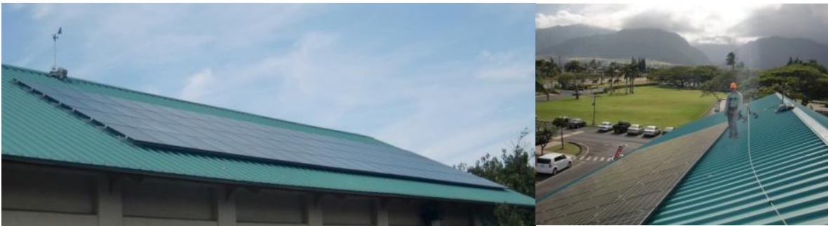
Figure 17: UHMC, Kahului, Maui – Roof mounted PV systems (left) on the north shore, four miles from the West Maui Mountain (right)
